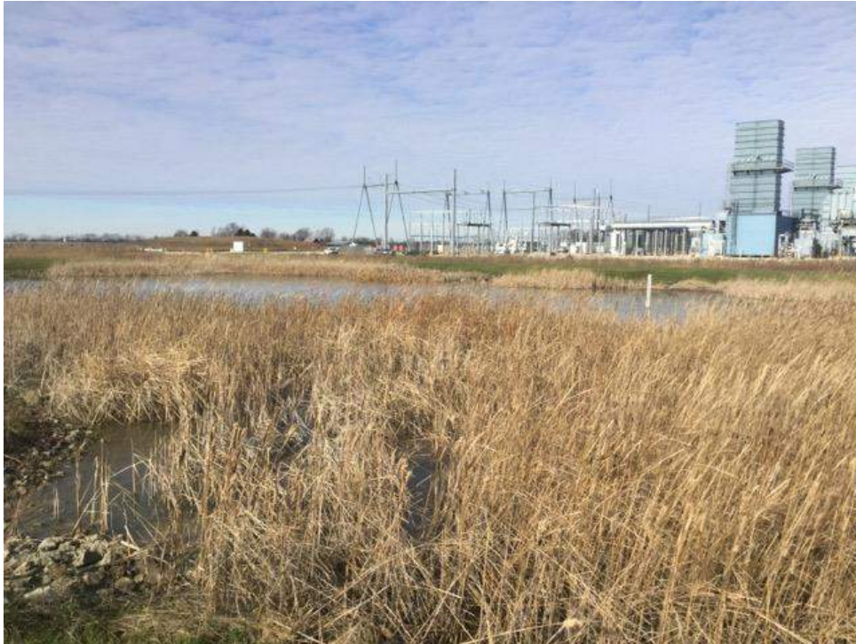
Photo Location 4. View of Open Water 1, storm water retention pond. Photograph taken facing northwest.
